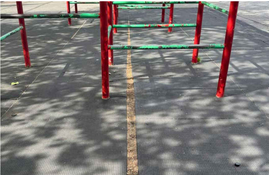
Gaps in safety surface
