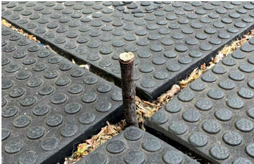
Gaps in safety surface
