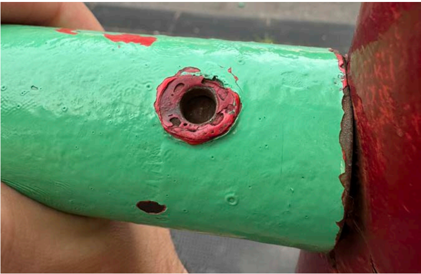
Missing bolt and rust
