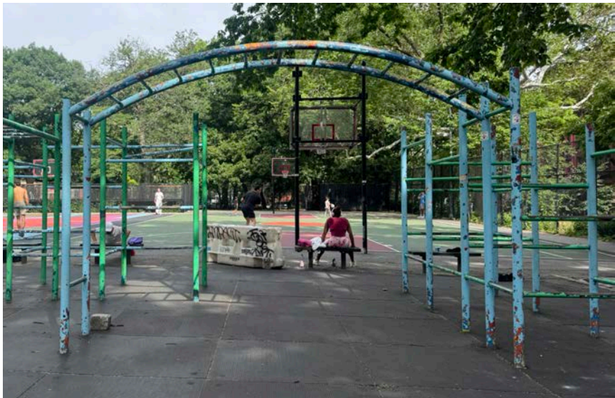
Fitness Blue Unit #2 with peeling paint
