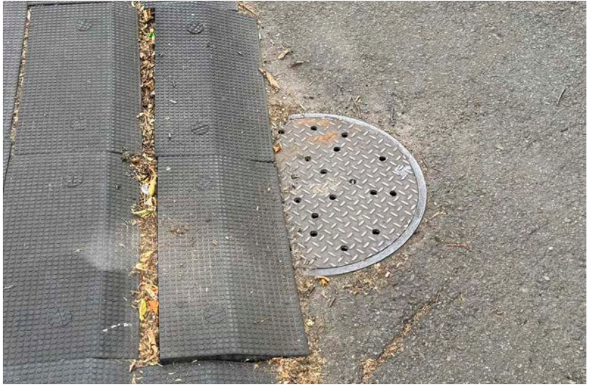
Loose, degrading safety surface tiles over manhole
