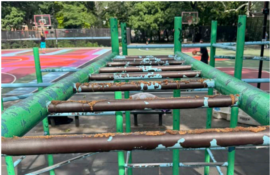
Debris on overhead ladder
