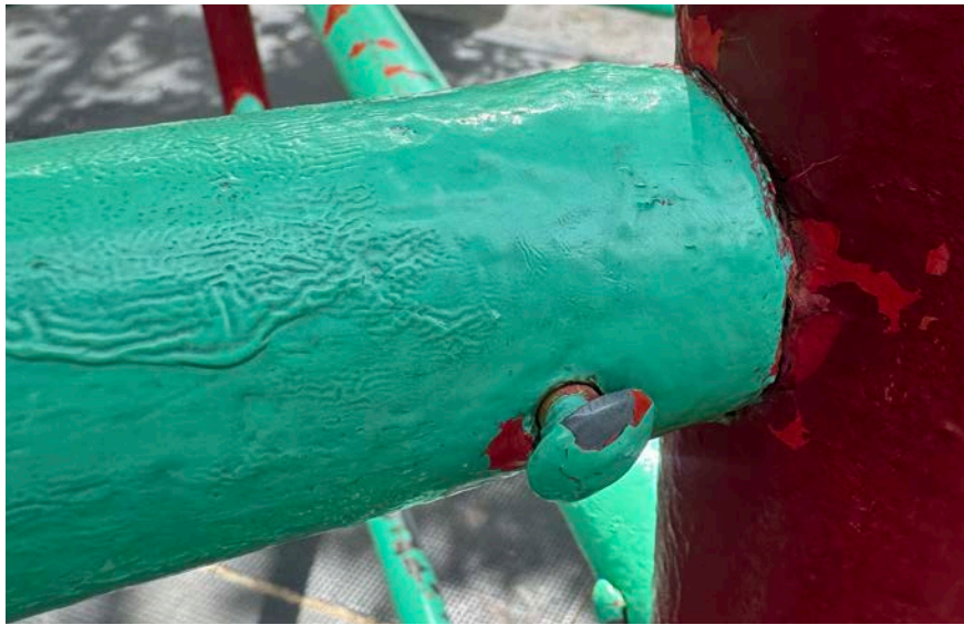
Loose bolt and entanglement hazard
